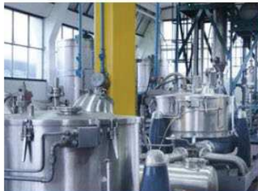
Package units and modular manufacturing
