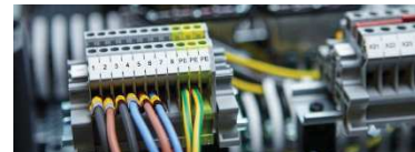
Control systems and distribution boards
